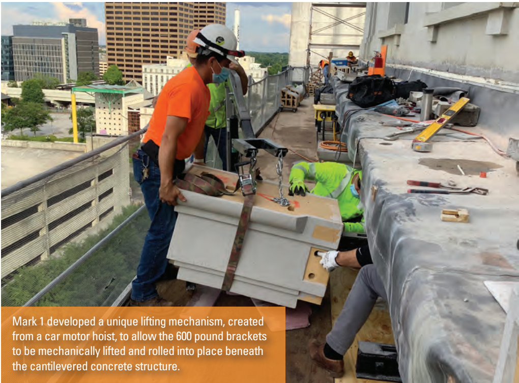
To save time and money, two of the terra cotta courses were extruded as one course with a false joint to replicate the appearance of the original cornice.
